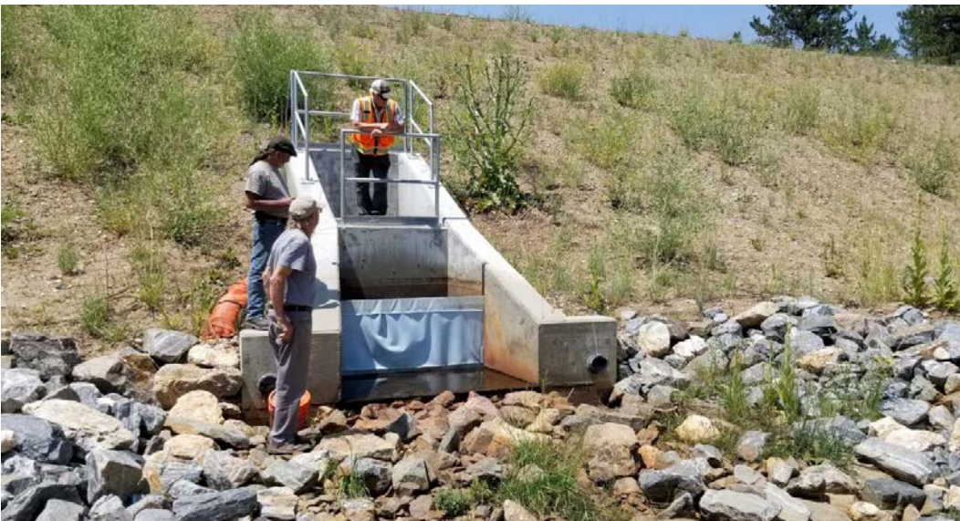
Photo of the outfall structure. Note screens on the toe drains should be replaced with larger mesh size.
