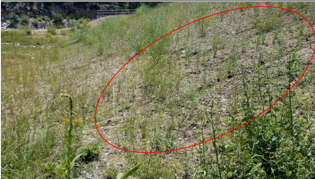
Photo of the erosion rills that are forming on the slope north of the outlet.
