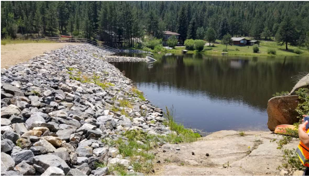
Typical photo taken along the upstream slope from the north end of dam looking south.
