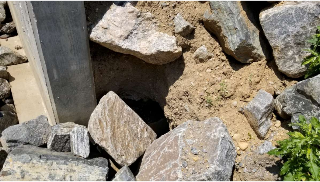
Photo showing the erosion occurring at the transition between the north training wall and riprap channel.
