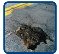
POTHoles/ DAMAGED PAVEMENT
