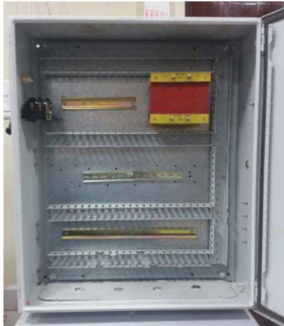
CONTROL PANEL WITH RACEWAYS/DIN RAILS
