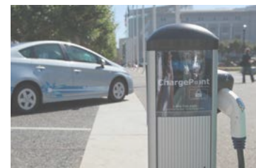
EV Charging Stations
