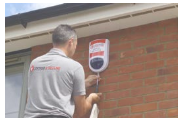
Security Alarm Systems
