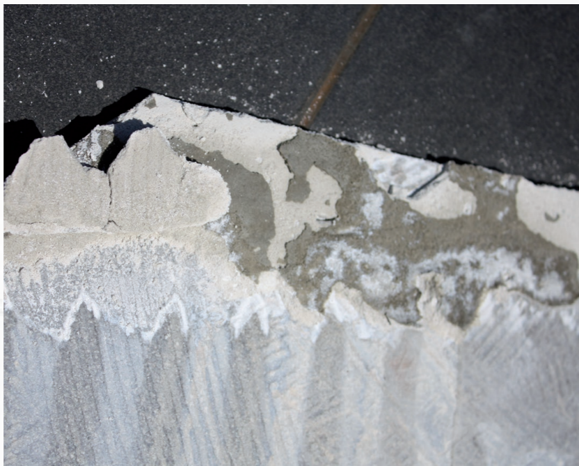
PHOTOGRAPH 5: This image shows adhesive on tiles in various states of final curing. The tile bonded around the edges strongly, then less well towards the centre where prolonged moisture content and slow setting has retarded the outcome. Poor trowel method has exacerbated this problem.
