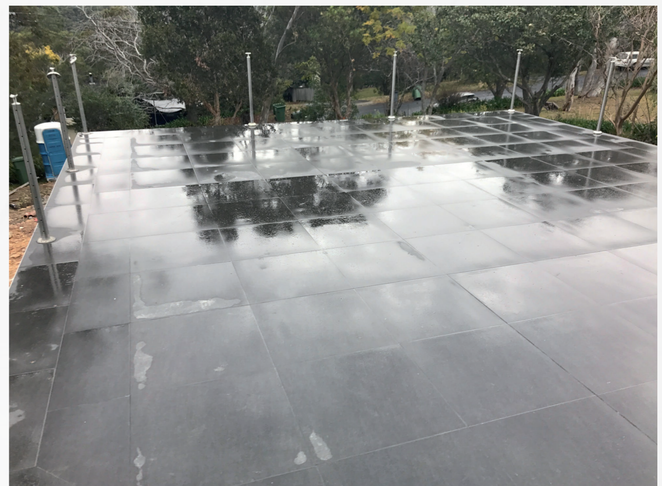
PHOTOGRAPH 6: This image shows external work exposed to rain during winter. Some joints aren't filled allowing ingress of water.
