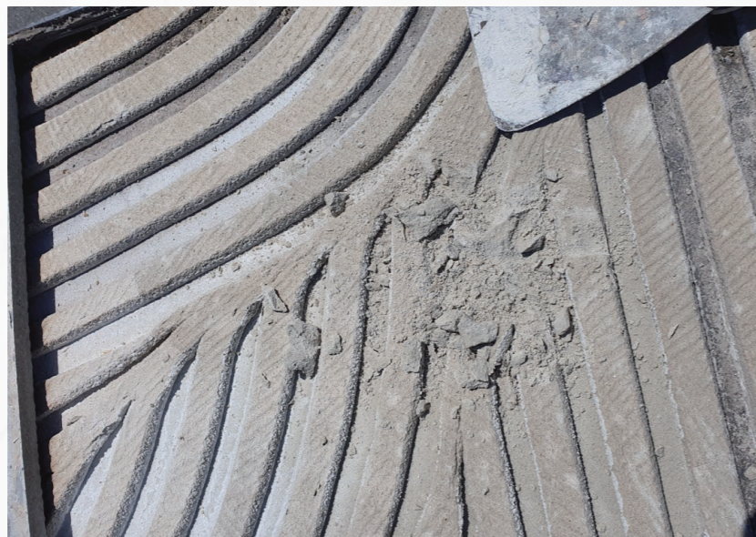
PHOTOGRAPH 4: This image shows degraded adhesive which is weakened and crumbling through lack adequate curing and moisture impact.
