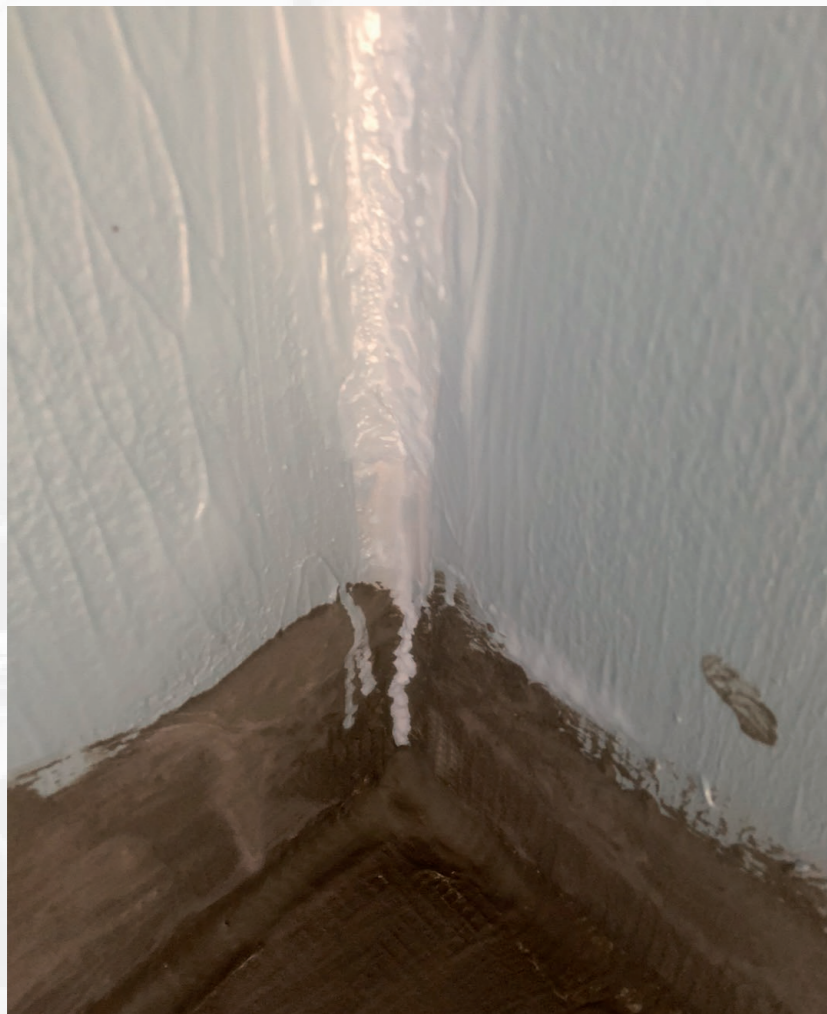
PHOTOGRAPH 1: This image shows a waterproofing membrane two days old, applied over a fillet bond breaker. The temperature is insufficient for curing of the membrane to take place. The membrane curing remains in a liquid state.
