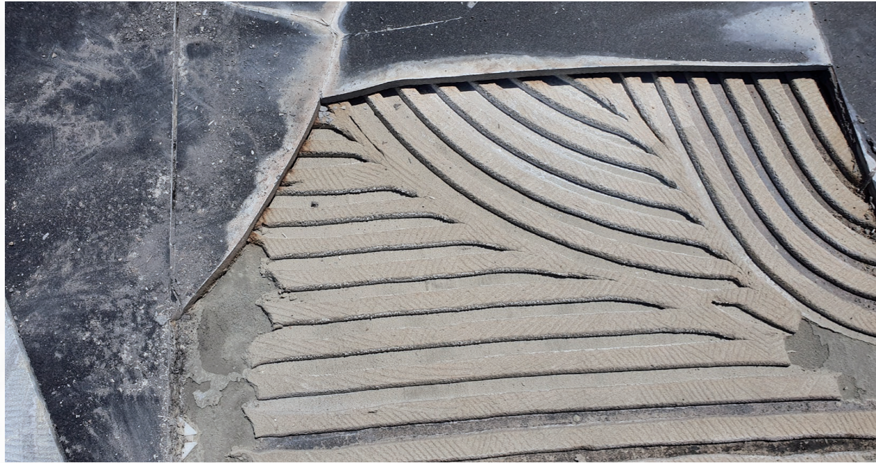
PHOTOGRAPH 2: This image displays lack of adequate bond in the centre of the tile. The trowel technique has added to the ability to retain moisture. The tiles are 600mm x 600mm. Installation was done directly to waterproofing membrane during winter in Sydney, Australia. There was rain on the installation and the average temperatures in the installation period range from a high of 18 degrees Celsius and average low is nine degrees Celsius
