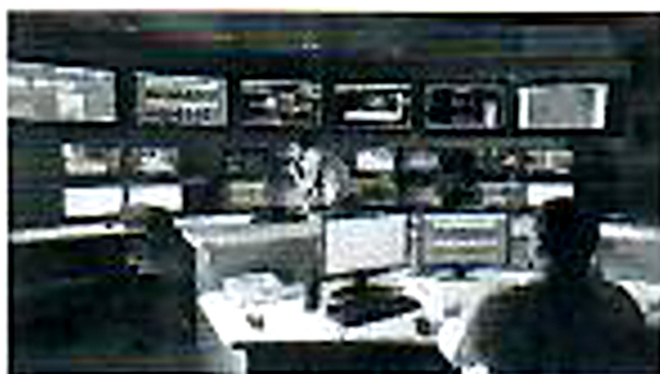
Command and control center
