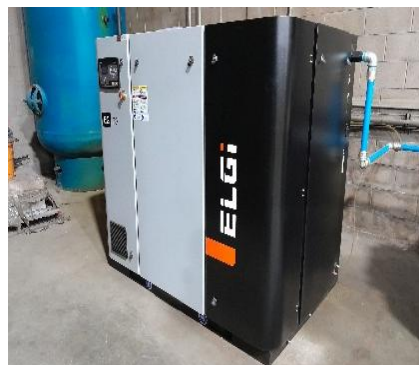
New VFD Air Compressors for Multiple KUKA Sites
