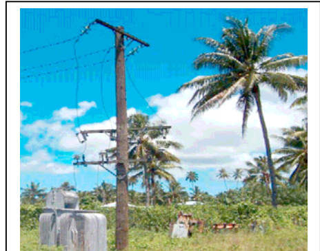
Figure 13: The viability of the use of coconut oil for electricity generation to supplement for diesel will be explored and assessed.
