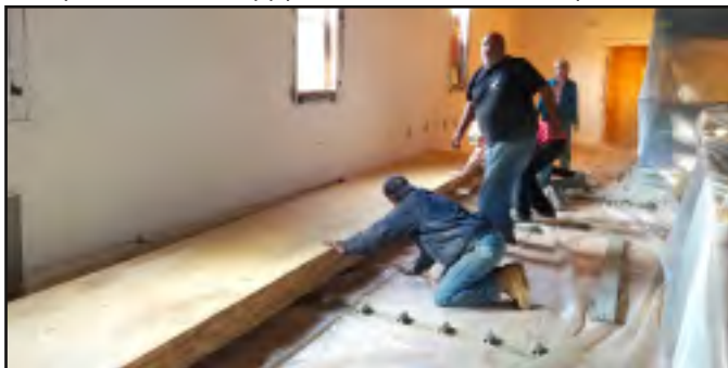
Progress! Friends help Brian wrestle the huge bar slabs into Burgee Dave's, as renovation goes forward. Photo - Kaitlyn Doorsi
