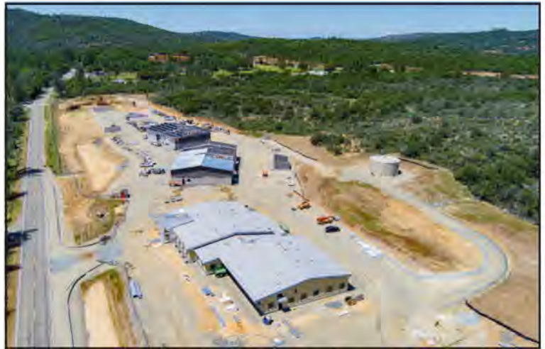
Work continues on Yuba Water Agency's new facilities on Marysville Road. All five buildings on the property are taking shape and work is on schedule.
