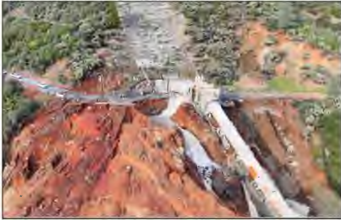
Site of Penstock Rupture (see p 6) Photo By Yuba Water
