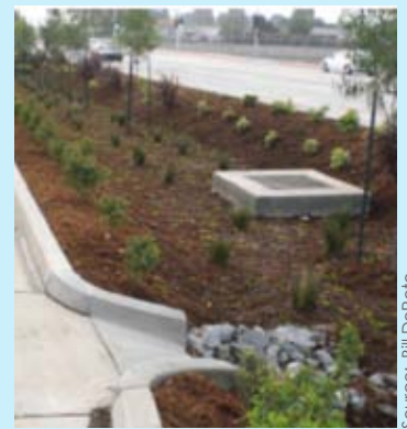
An overflow outlet conveys runoff that exceeds the bioretention area capacity.
