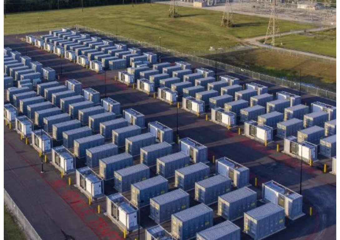
One of Jupiter Power's operational battery energy storage systems in Houston
