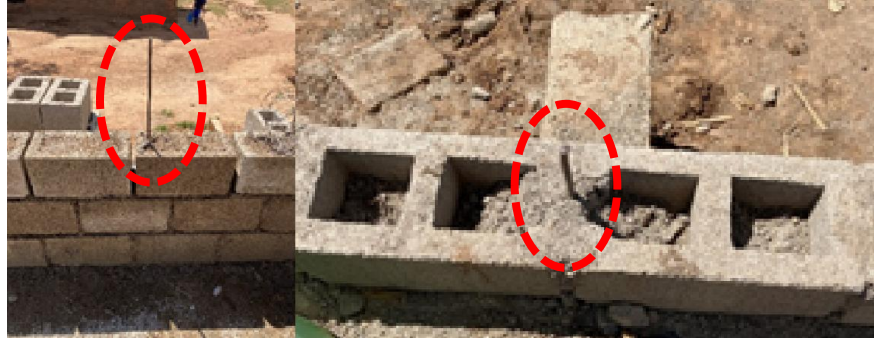
Figure 4. Examples of improperly placed vertical rebar
