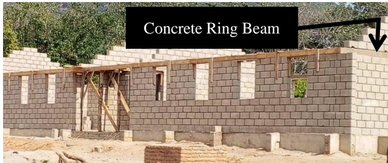
Figure 5. Concrete ring beam depth is not 300 mm, but rather 200 mm
