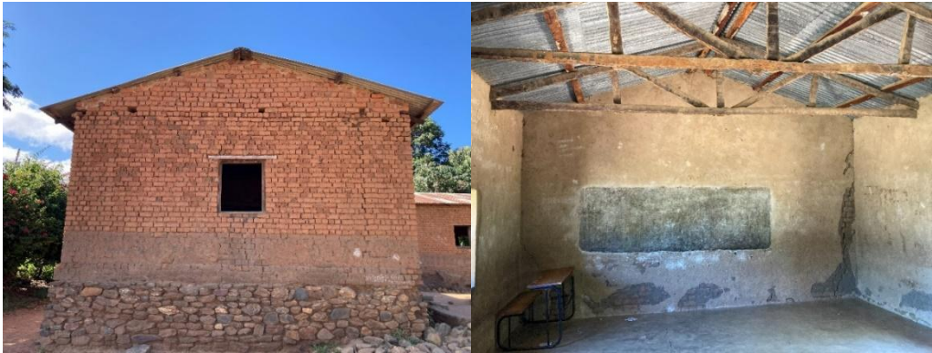
Figure 1. Deteriorated exterior and interior condition of the 1940s school building
