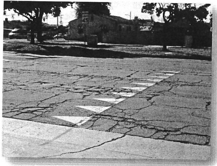
Figure 2: Alligator Cracking along Central Avenue
