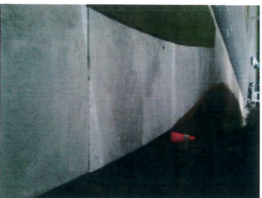
1 to 1 1/2 Inches High Repair by Precision
