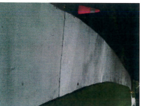
1 1/2 to 2 Inches High Repair by Precision
