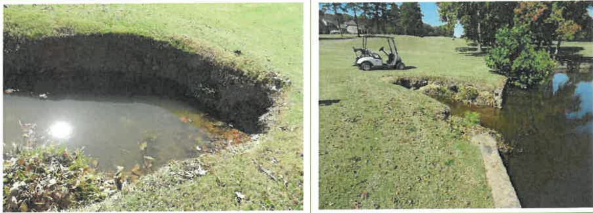
Images of the lake-bank by hole #9 that has been impacted by runoff, which could continue to get worse if not addressed.
