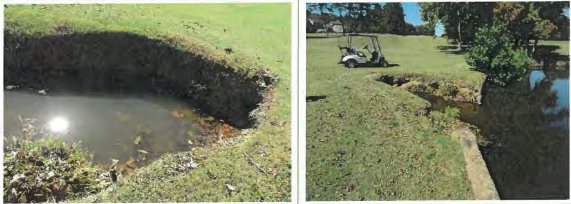
Images of the lake-bank by hole #9 that has been impacted by runoff, which could continue to get worse if not addressed.
