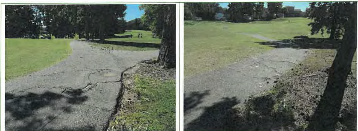
Images of cart paths at JPGC showing the uneven surface and the impact of tree roots. This condition can make the ride in carts uncomfortable for players and leads to driving on grass causing other damage. Paths like this also add to the wear and tear on carts.
