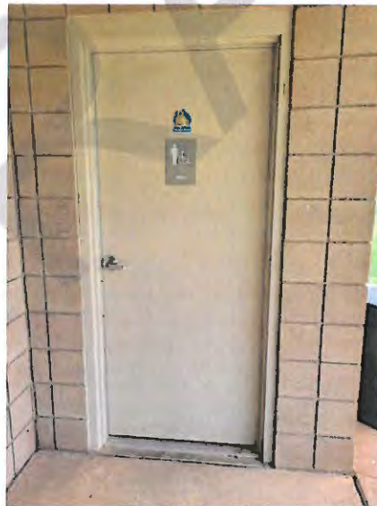
Figure 69: Jamestown Soccer Fields Men's Toilet Room Door
