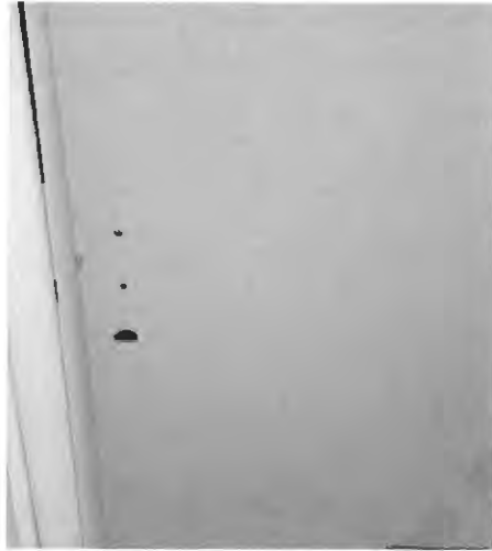
Figure 32: Jamestown Fire Station Men's Toilet Room Door
