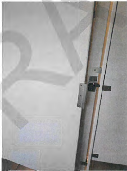
Figure 17: Jamestown Civic Center Toilet Room Door Hardware
