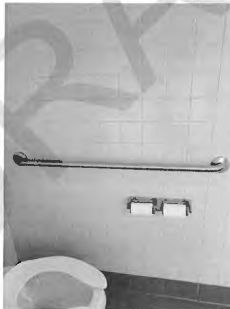
Figure 15: Jamestown Civic Center Toilet Room Grab Bar
