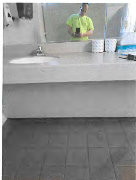
Figure 12: Jamestown Civic Center Toilet Room Lavatory
