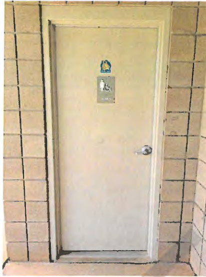
Figure 70: Jamestown Soccer Fields Women's Toilet Room Door
