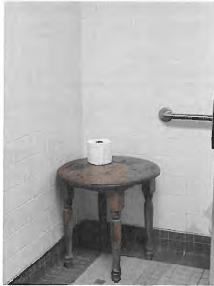
Figure 24: Jamestown Fire Station Men's Toilet Room Obstruction
