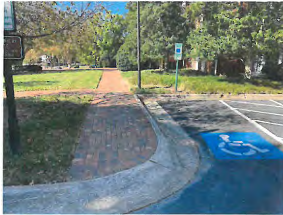
Figure 36: Jamestown Library Inaccessible Route
