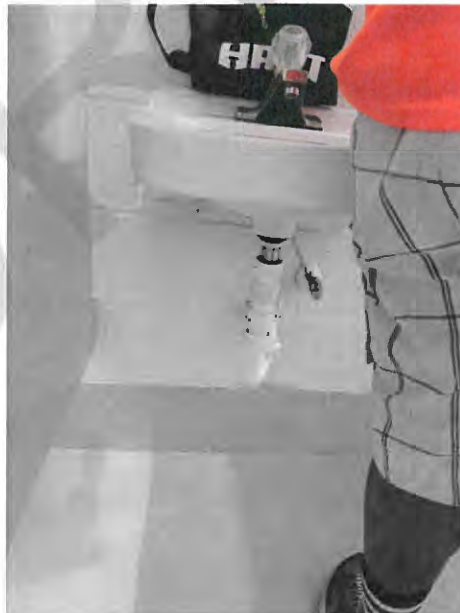
Figure 62: Jamestown Public Park Bathroom Sink View 1
