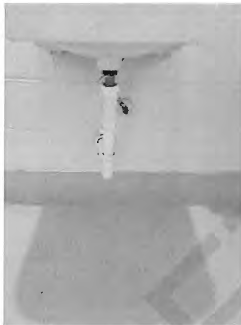
Figure 63: Jamestown Public Park Bathroom Sink View 2
