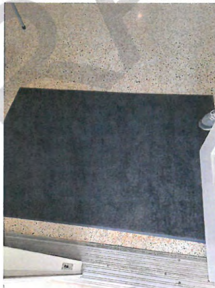
Figure 81: Jamestown Town Hall Door Threshold
