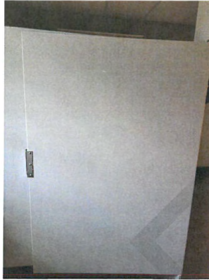
Figure 16: Jamestown Civic Center Toilet Room Door
