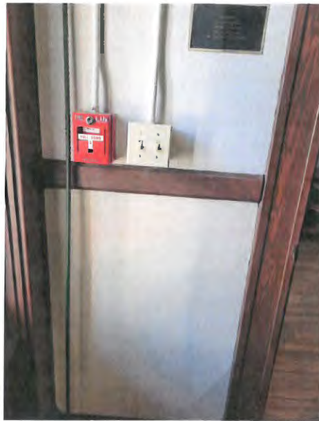
Figure 41: Jamestown Library Light Switch
