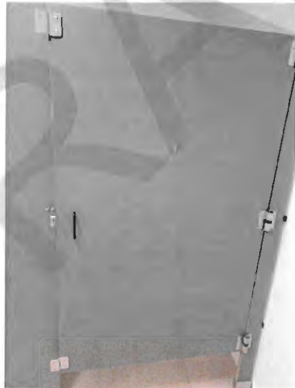
Figure 73: Jamestown Soccer Field Toilet Room Stall Door
