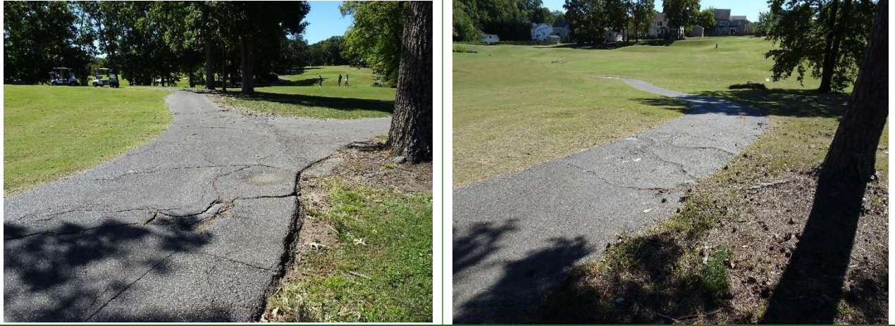
Images of cart paths at JPGC showing the uneven surface and the impact of tree roots. This condition can make the ride in carts uncomfortable for players and leads to driving on grass causing other damage. Paths like this also add to the wear and tear on carts.
