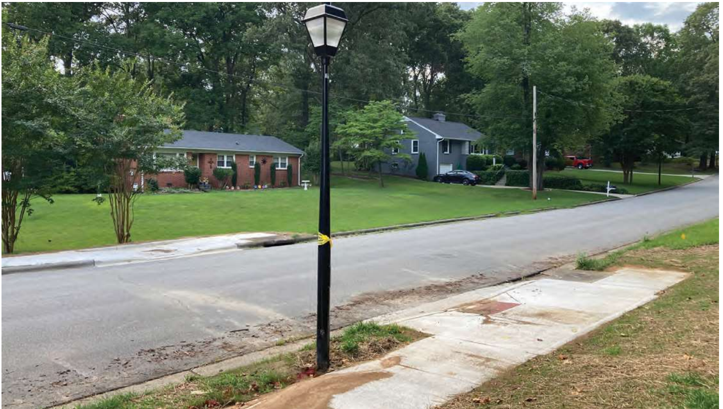
A newly constructed sidewalk on Potter Drive is the latest addition to Jamestown's growing pedestrian network.
