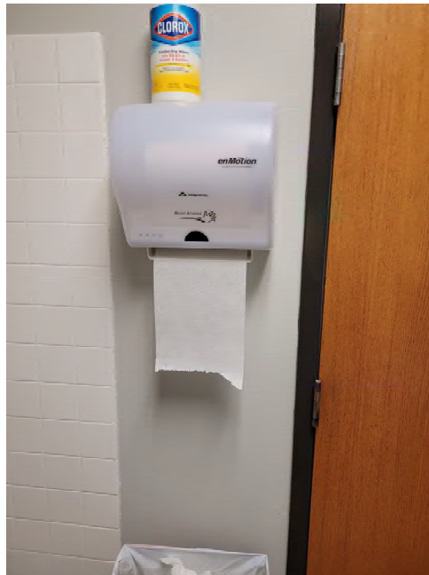
Figure 29: Jamestown Fire Station Men's Towel Dispenser
