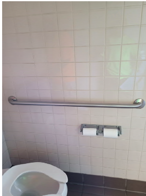
Figure 15: Jamestown Civic Center Toilet Room Grab Bar
