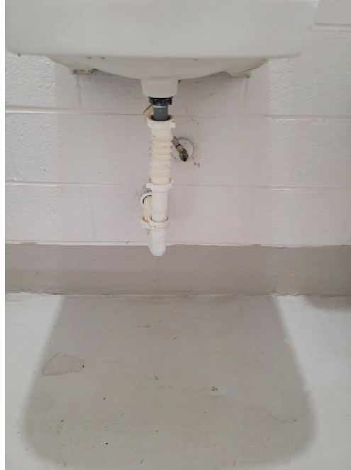
Figure 63: Jamestown Public Park Bathroom Sink View 2
