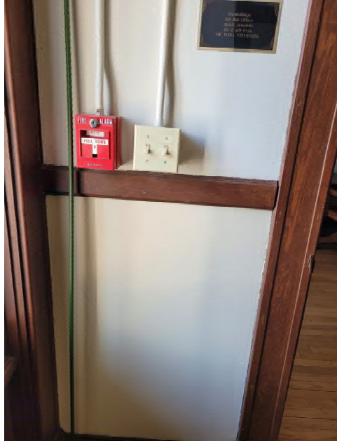
Figure 41: Jamestown Library Light Switch
