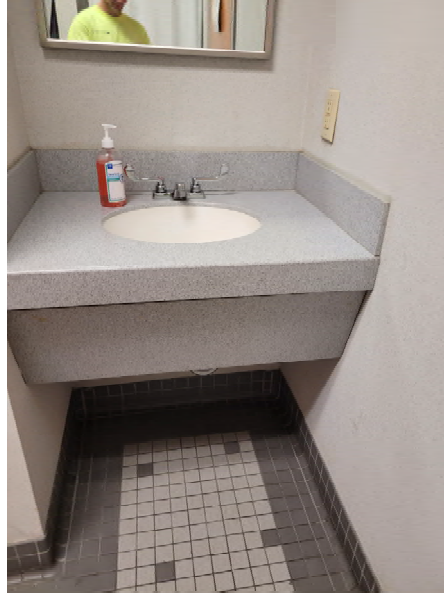
Figure 28: Jamestown Fire Station Women's Toilet Room Sink
