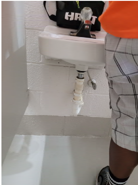
Figure 62: Jamestown Public Park Bathroom Sink View 1
