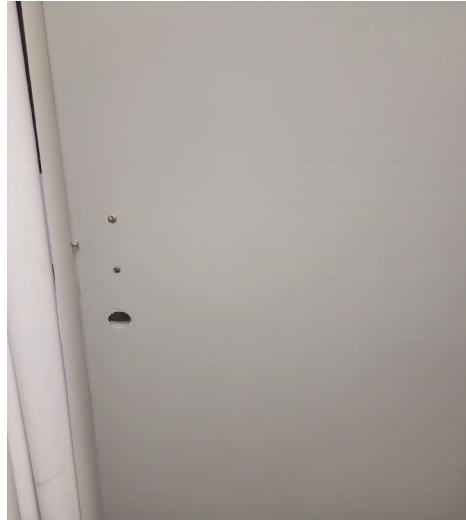
Figure 32: Jamestown Fire Station Men's Toilet Room Door
