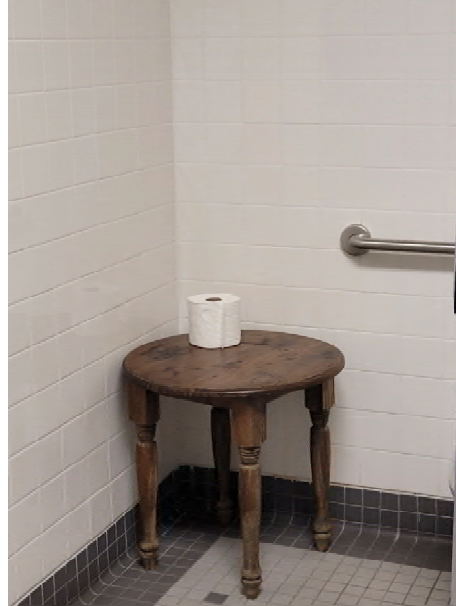
Figure 24: Jamestown Fire Station Men's Toilet Room Obstruction
