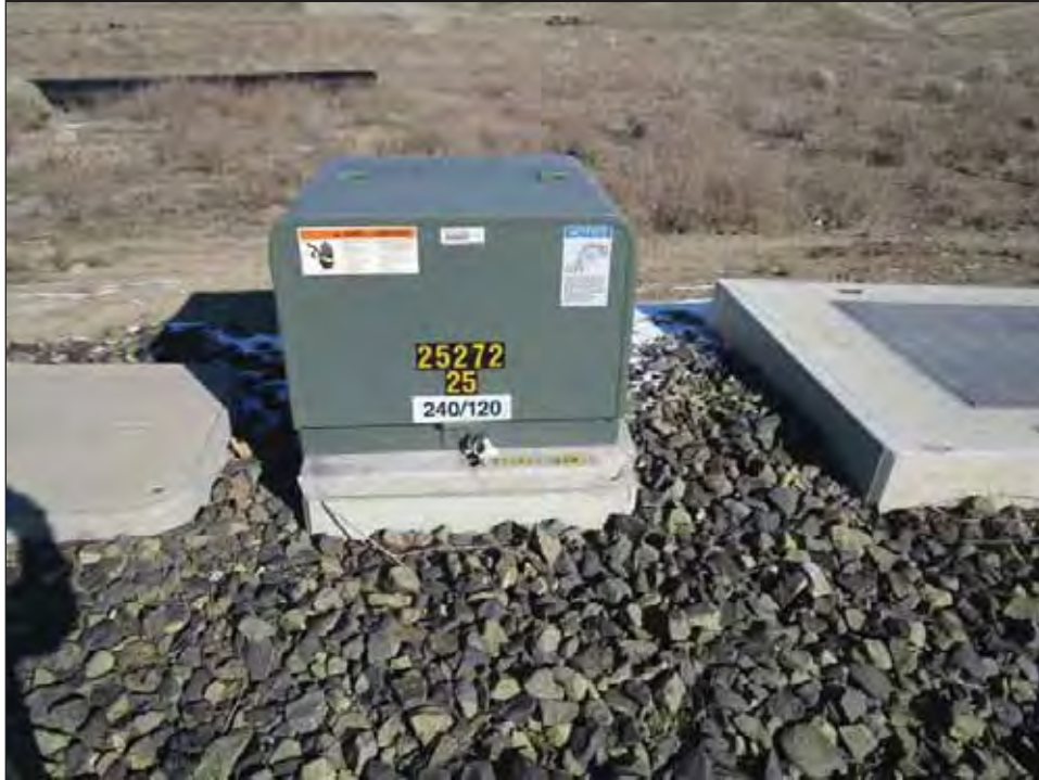
Photo 10: Pad mounted transformer
