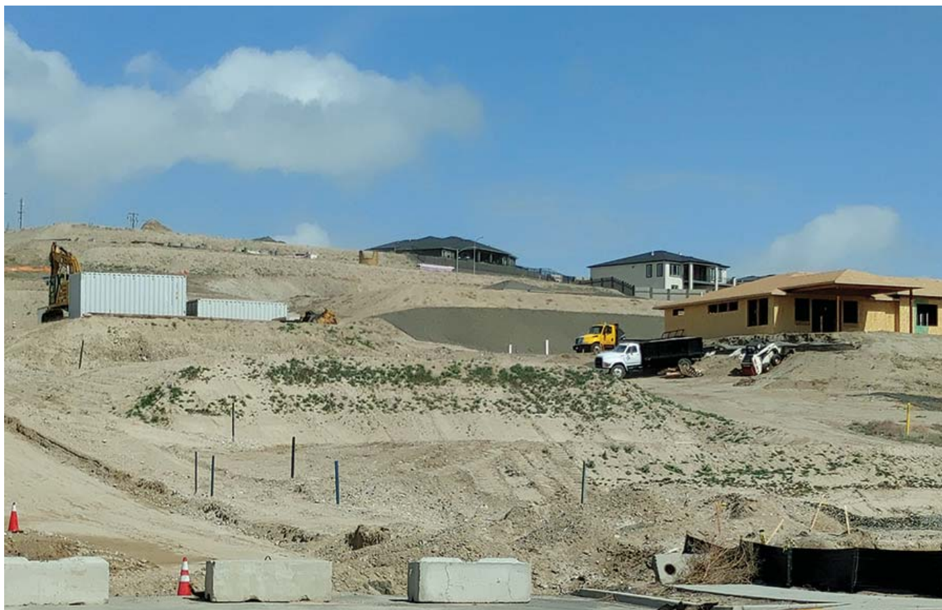
( https://4aai724b033c18zdidiy/gmgw/markin/Bob/Chris/Parckway.jpg ) Developers terrace home sites on the south side of Thompson Hill, near Kennewick's Southridge High School. (Photo by Wendy Culverwell) ( https://4aai724b033c18zdidiy/gmgw/markin/Bob/Chris/Parckway.jpg )
