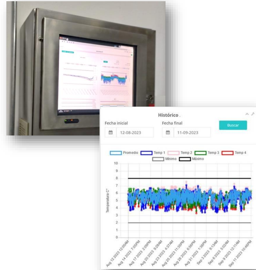
Telemetry system with remote monitoring (since 2010)
