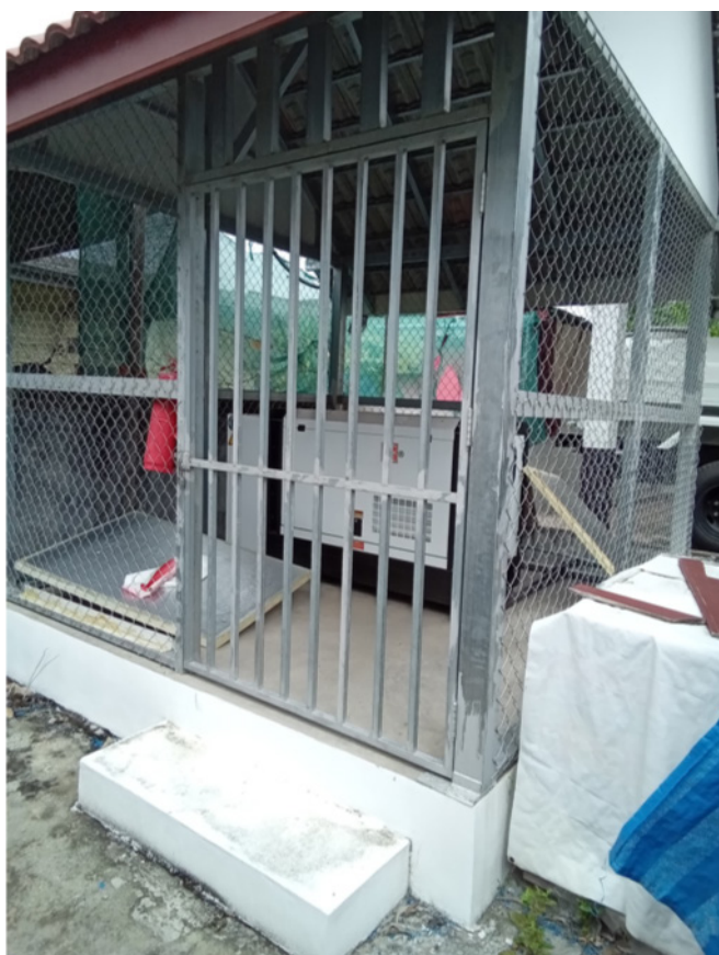
Figure 20: Secure generator housing at Luang Prabang Provincial Vaccine Store
