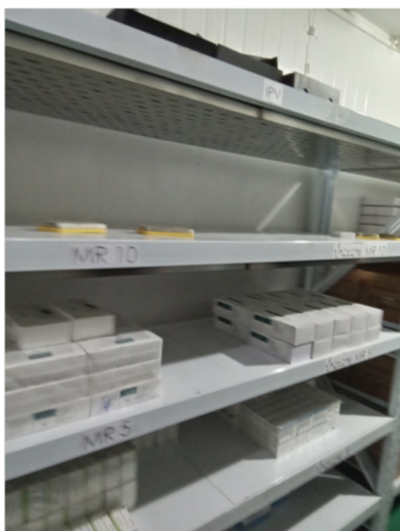
Figure 18: Vaccines are stored by type in walk-in cold room at Champasak Provincial Vaccine Store
