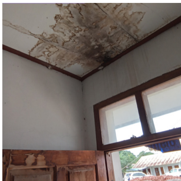
Figure 28: Poorly maintained ceiling at a health centre in Phongsaly
