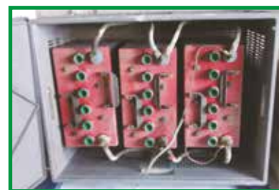
Battery Bank of Solar Refrigerator
