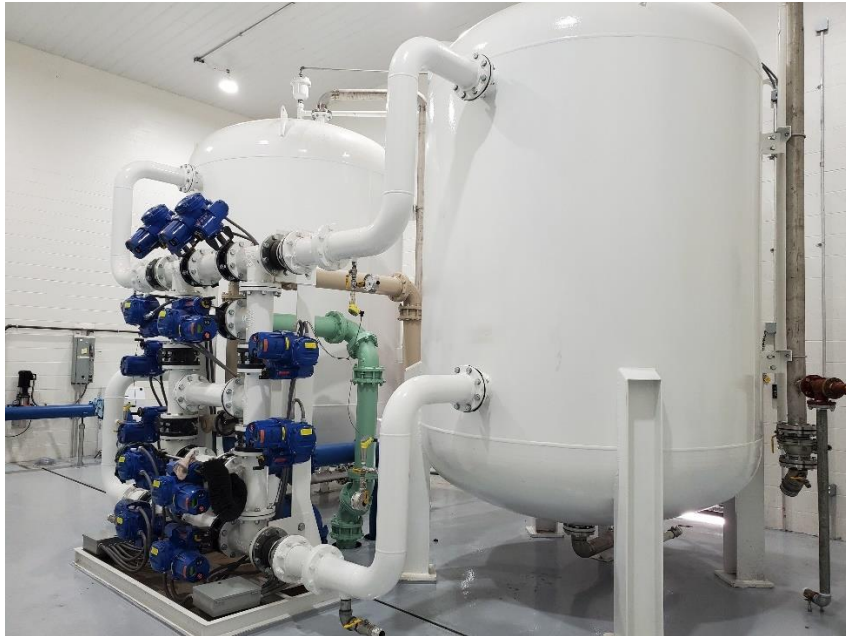
GAC treatment system constructed in Warrington Township for the North Wales Water Authority
