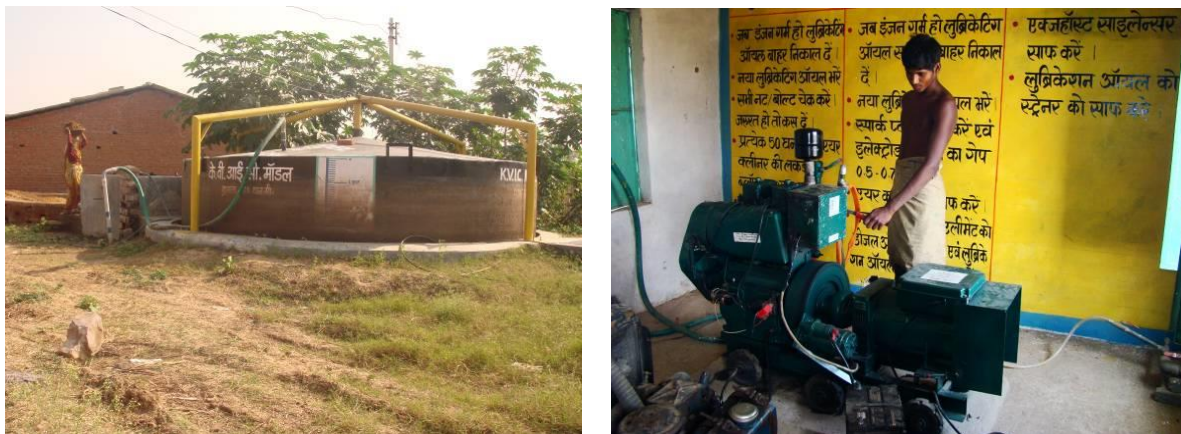
Figure 3. Biogas plant and generator to produce electricity
