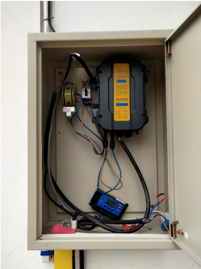
Power converter and controller.
