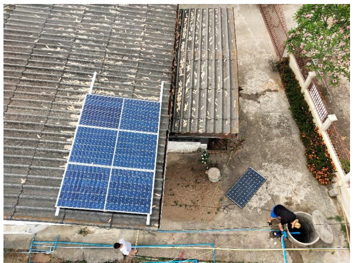
Roof mounted Solar Panels.
