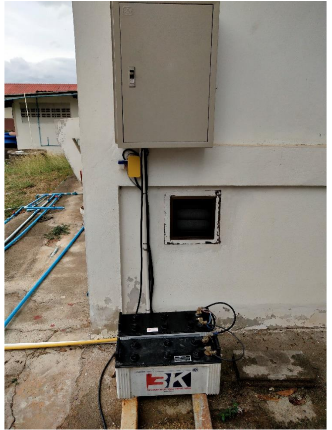
Batteries and switch board.
