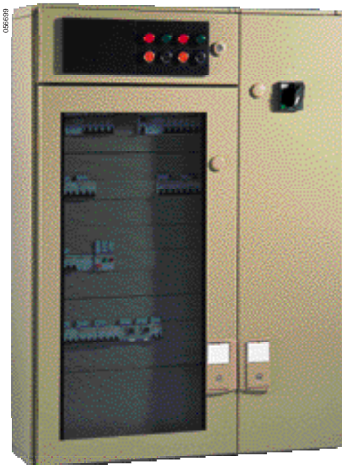
Power distribution incomer in a Prisma GK cubicle
