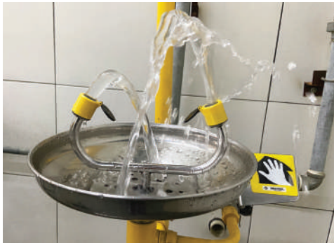
Occasional unbalanced water stream
