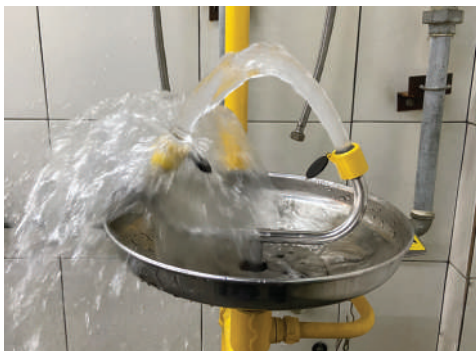
Unchecked pressure leads to messy and wet surroundings
