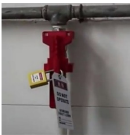
Locked with opened valve
