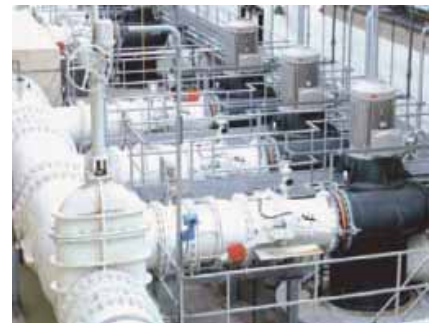
Reliability of operation through years of experience
