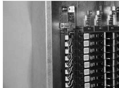
FIGURE 8. BREAKERS CONNECTED TO BCB
