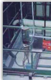
Gravity feed oiler on drying machine
