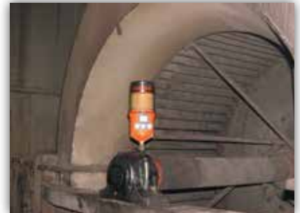
Grease lubricator installed on a blower fan
