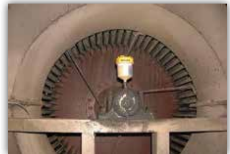
Streamliner V installed on a blower fan
