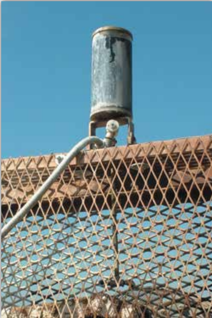
Chain oiler lubricating a chain on a trommel screen
