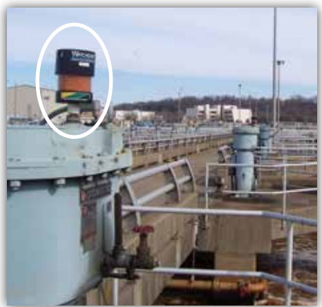
Watchdog Breather installed on a gearbox at a water treatment facility
