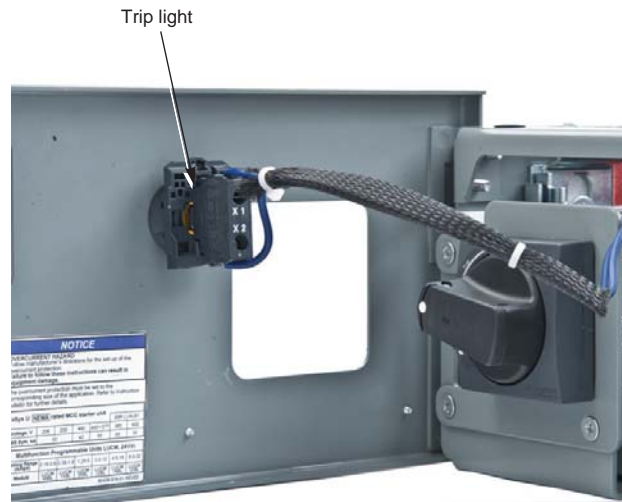
Figure 18: Trip Light (Back of Door)
