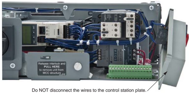
Figure 25: Control Station Plate (Removed)
