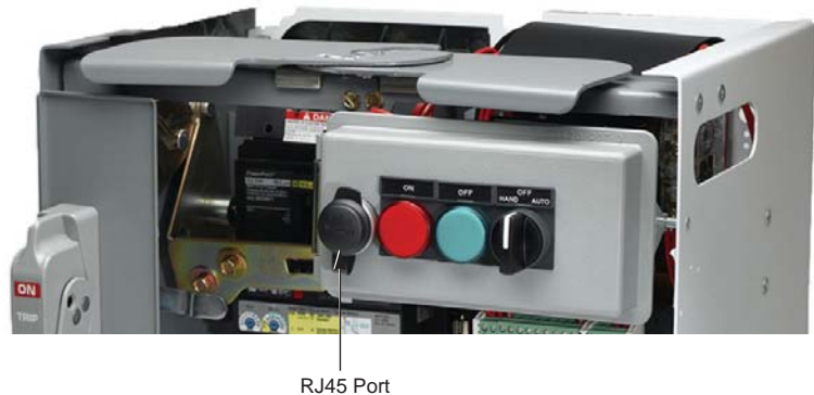
Figure 11: Location of RJ45 in NEMA 12 MCC Enclosures
