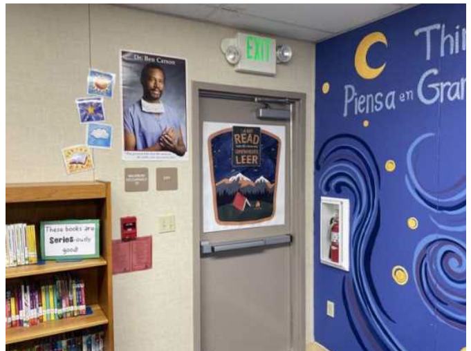
22 - FIRE ALARM COMPONENTS
