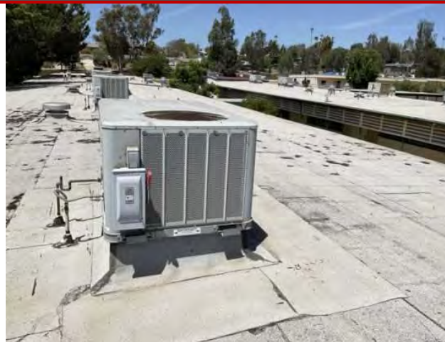
14 – ROOFTOP PACAKAGED UNITS
