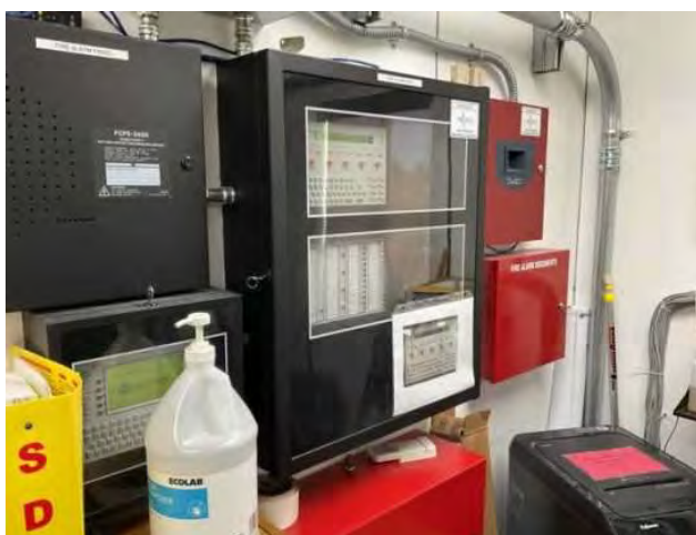
17 - FIRE ALARM PANEL
