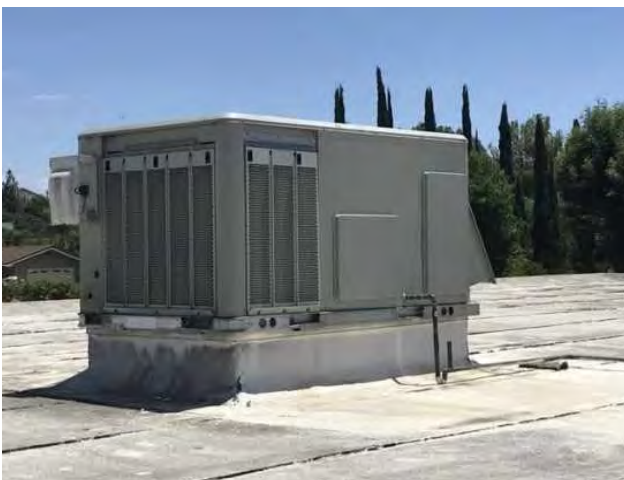
29 - ROOFTOP PACKAGED UNIT
