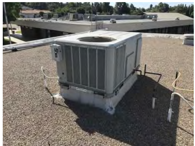
30 - ROOFTOP PACKAGED UNIT
