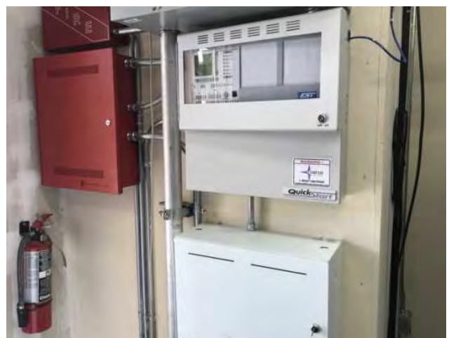
36 - FIRE ALARM PANEL
