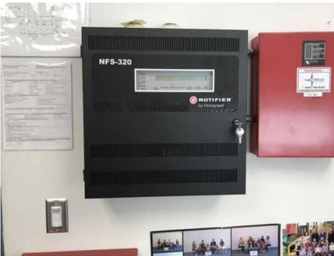
27 - FIRE ALARM PANEL
