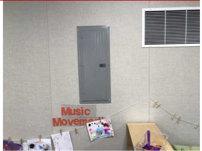
26 – ELECTRICAL DISTRIBUTION PANEL
