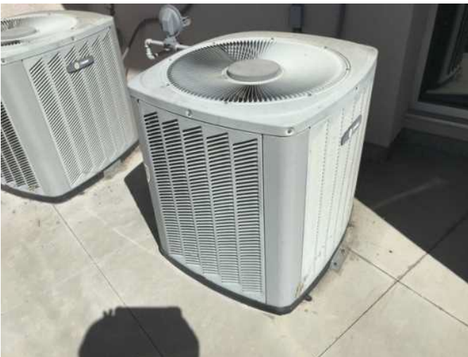
21 - SPLIT SYSTEM CONDENSING UNIT
