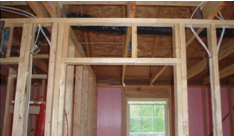
Ceiling trusses designed to span entire home. There are no bearing walls for the roof in the interior of the home. Duct shown is the fresh air intake for the house.
