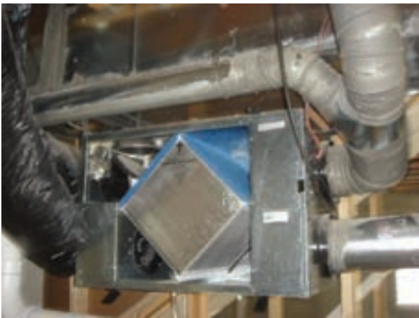
HRV ducted wet rooms
