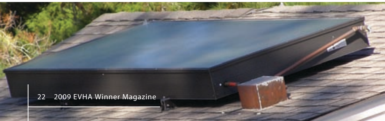
Solar water panel
