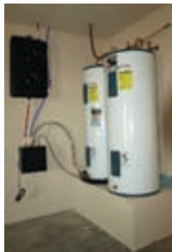
Storage and auxiliary water tanks for solar hot water
