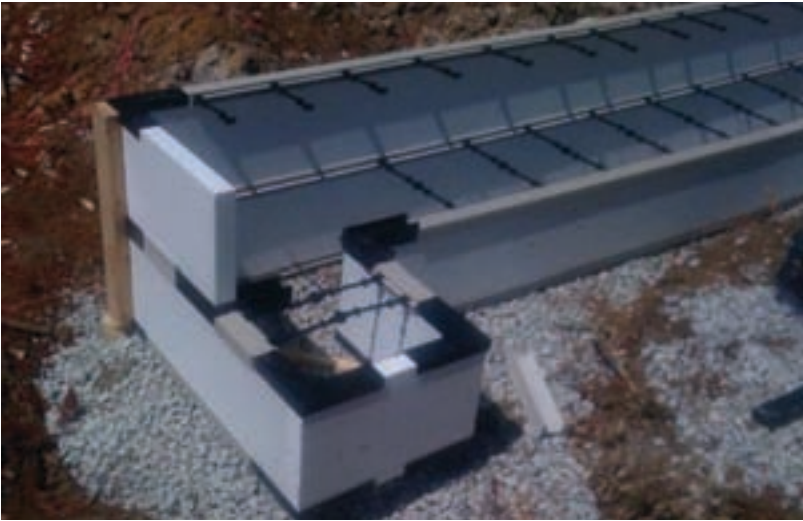
ICF foundation system, frost protected shallow foundation, foundation depth 12", 1" EPS foam under entire slab
