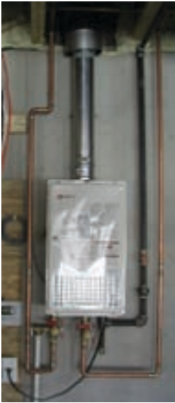
On-demand hot water heater
