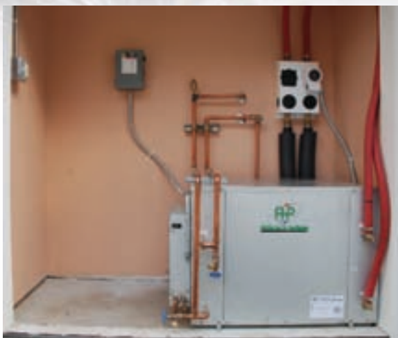
Insulated and sound-proofed heat pump closet
