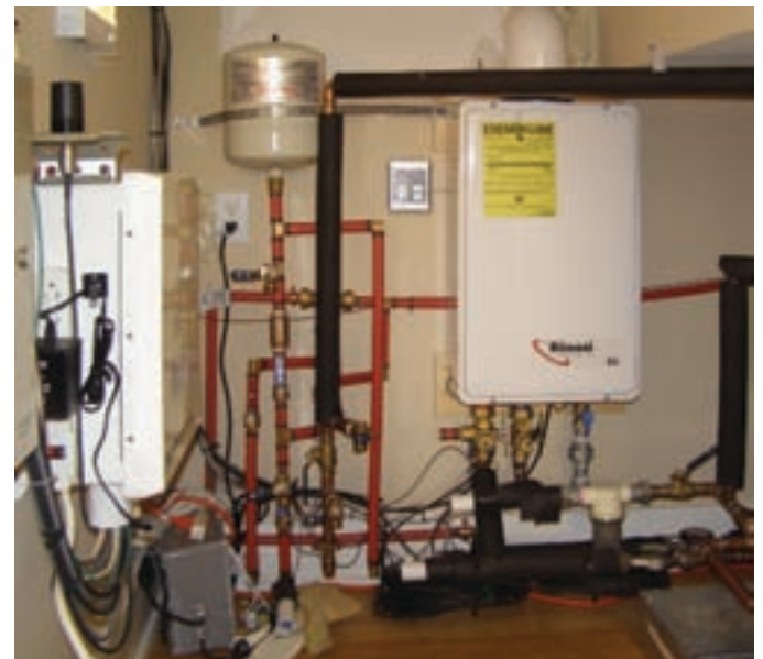
Tankless water heater and valving
