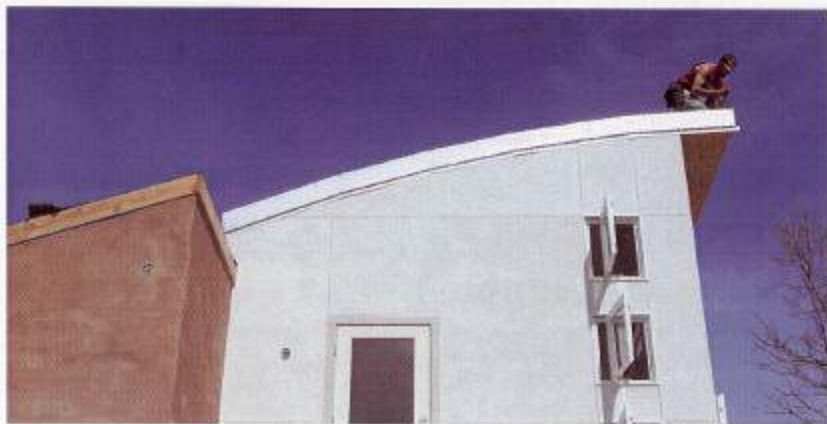
Brock Waits installs a metal roof on Heather Ferrier's energy-efficient house near Lake Weatherford.
