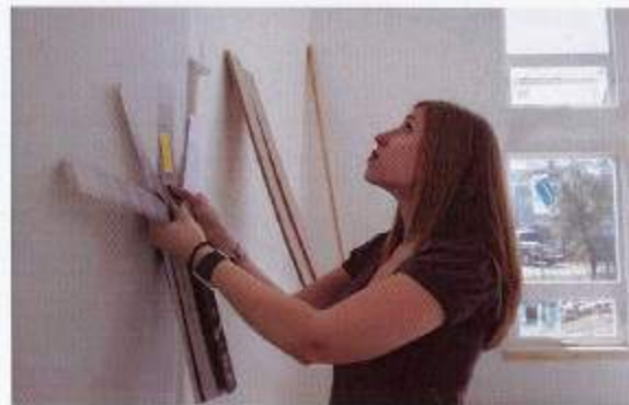
Most of the walls will be covered with white paint, which has the fewest harmful volatile organic compounds.
