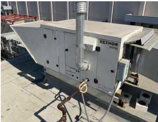
27 - MAKE-UP AIR UNIT
