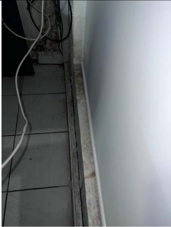
Continuous water leakage through the wall and first floor slab
