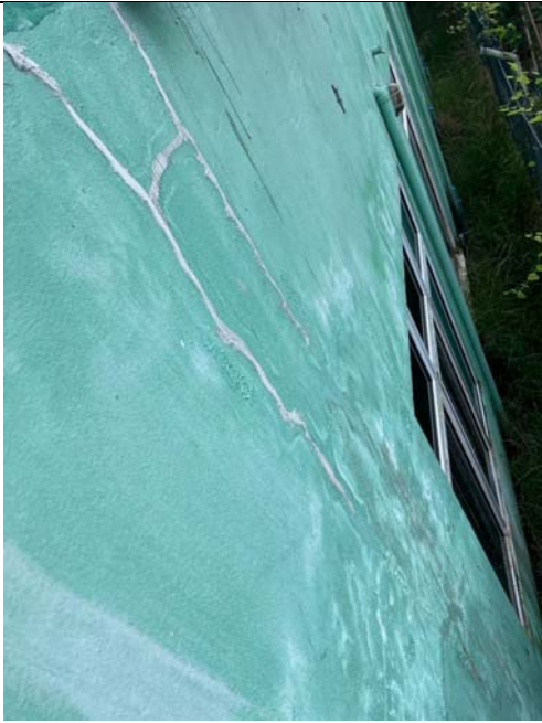
Damped exterior wall
