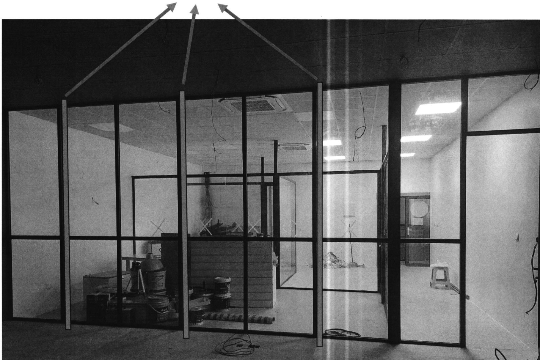
Fixing Galvanized Iron Hollow Pipes (Square) to Aluminum Partition as a Support.
