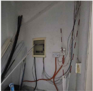
STORAGE ROOM - DB LOCATION
