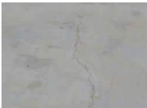
Fig 1. Cracks on Substrate
