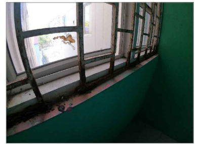
Replace all rusted grills
