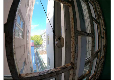
Replace all broken window handles
