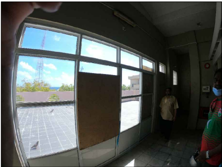
Fix all broken doors and windows
