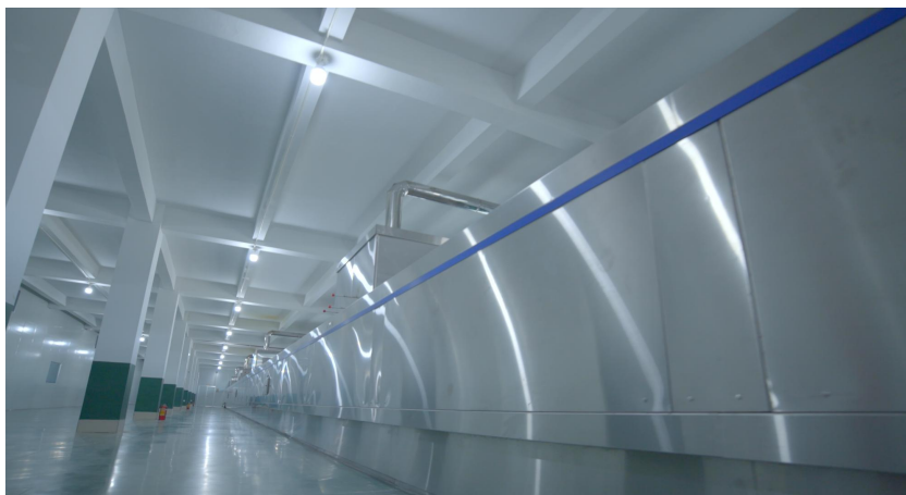
隧道炉 tunnel stove
