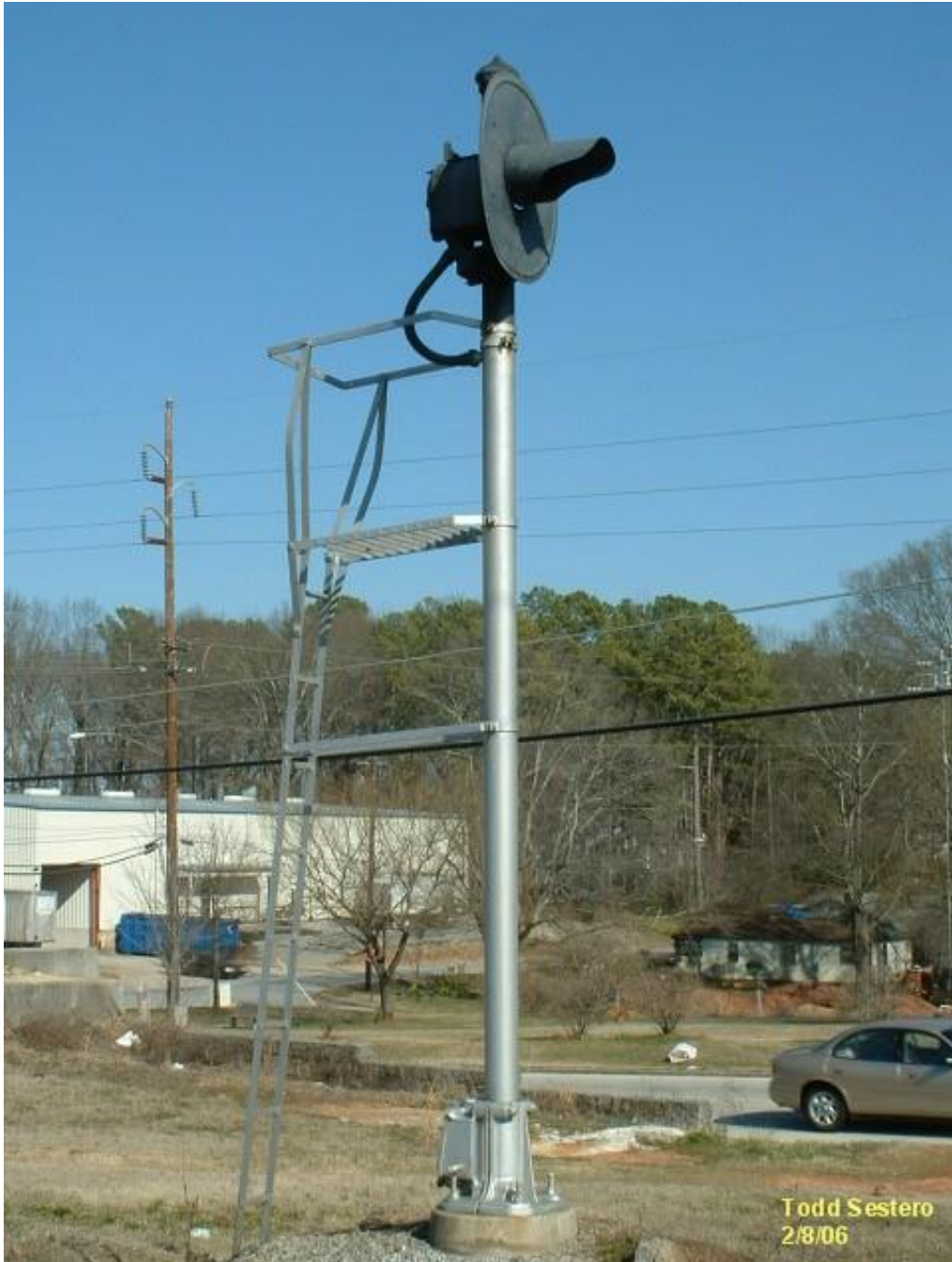
A couple of classic searchlight signal installations at the same location in suburban Atlanta, these are of the US&S variety. The easiest way to tell is by the hoods.
